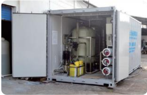
120tons \ day seawater desalination equipment Fiery Cross Reef in the South China Sea
