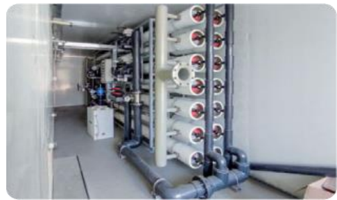
3840tons \ day seawater desalination equipment Xiamen
