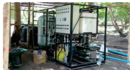
50tons \ day seawater desalination equipment Maldives
