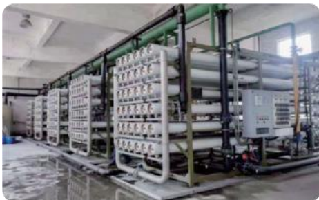
13000tons \ day seawater desalination equipment Malaysia
