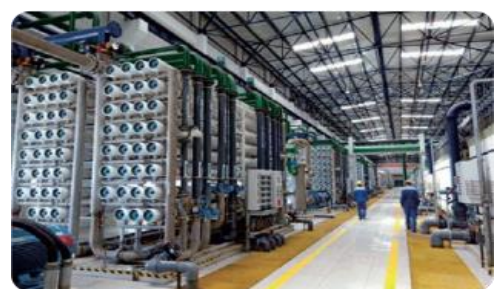
19000tons \ day seawater desalination equipment Malaysia
