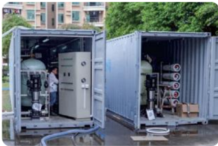
360tons \ day seawater desalination equipment South China Sea islands
